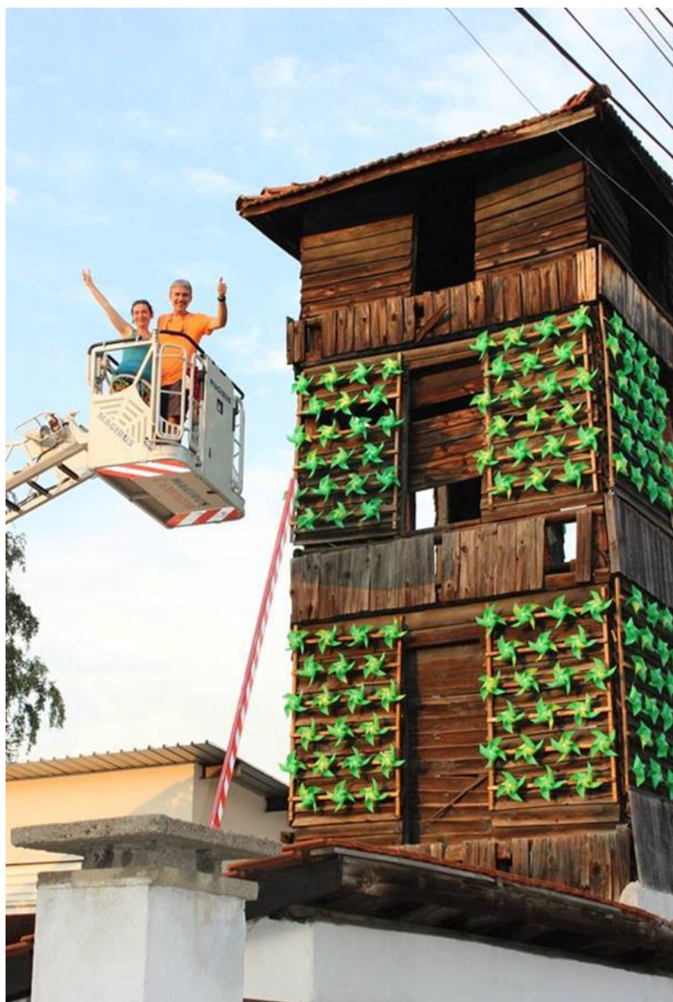
The process of the building of the kinetic installation “Breathe” – the fireman’s tower in Samokov, author: Hristo Gelov, august 2017.
